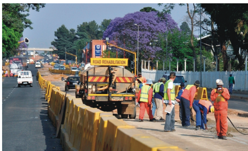
Figure 4: Road rehabilitation and maintenance are the key issues to maintain the quality of the road network. Photo by Carlos F. Pardo, Johannesburg, 2010
